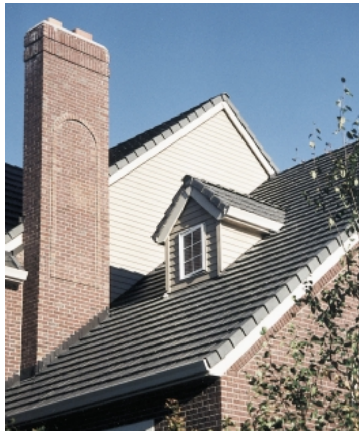
FIGURE 20.31 ■ Dormers allow windows to be added to attic areas. Courtesy LeRoy Cook.
