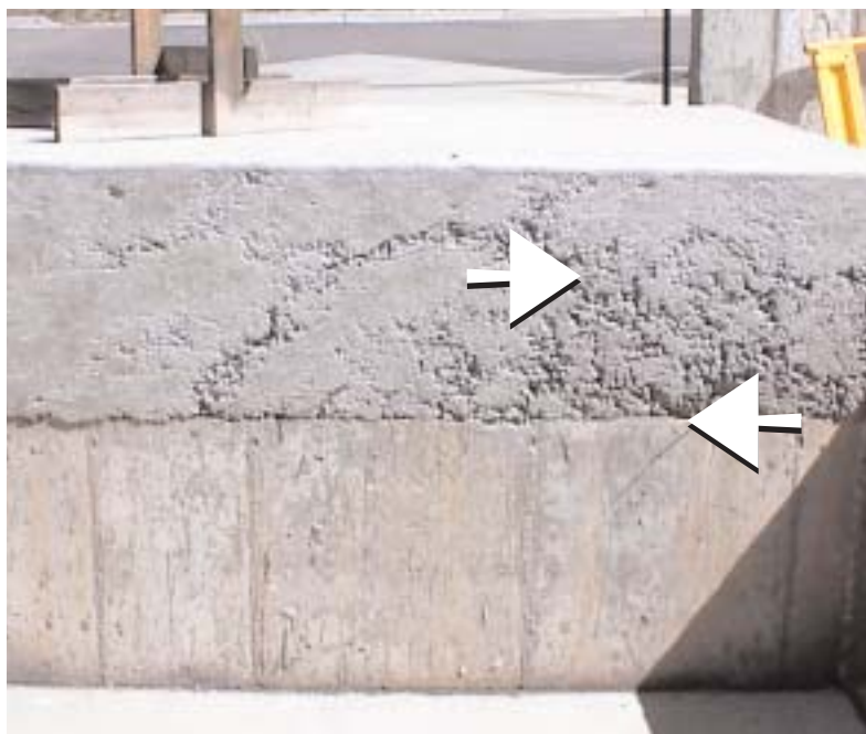
1-24 Cold joint (middle) with rock pockets (above)
