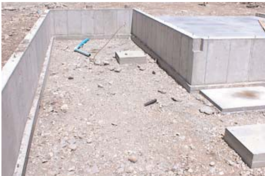
1-02 Soil, climate, and the weight of the house dictate the type of foundation used. Shown here is a perimeter wall on spread footing.
