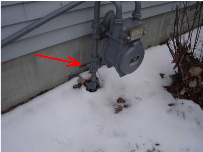
FYI - main gas line shut off on east side of home.
