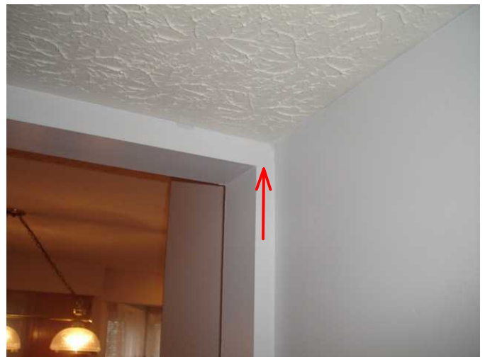
17) Settlement cracks in multiple areas. This is located in entry hall. Suggest repair and monitor.
