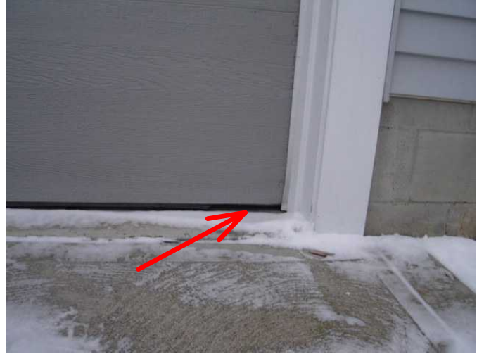
7) Door seal on bottom of garage door is damaged and may allow pests into the structure.
