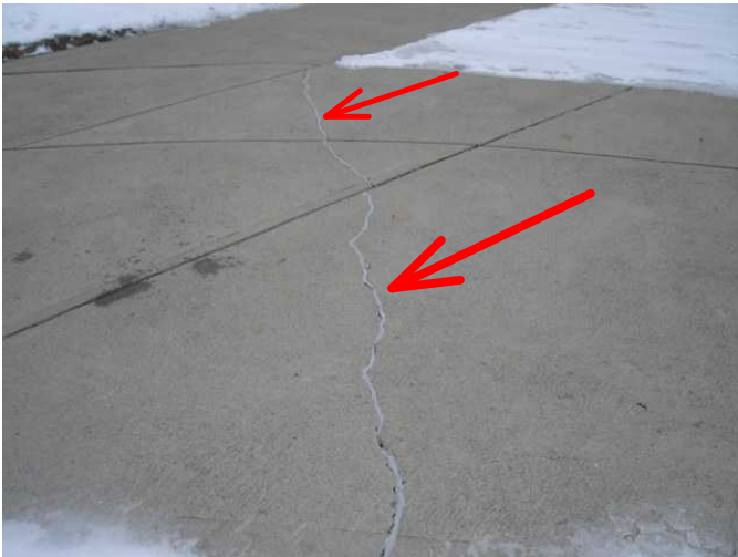
8) Settlement crack in concrete driveway. Monitor for movement and displacement.
