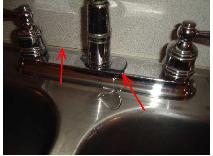
Caulking deteriorated at counter top / backsplash seam. Kitchen faucet leaks at base during operation.
