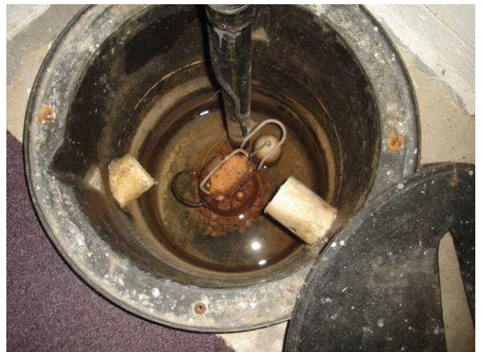
22) Sump pump operated but is rusted. Periodically test operation.
