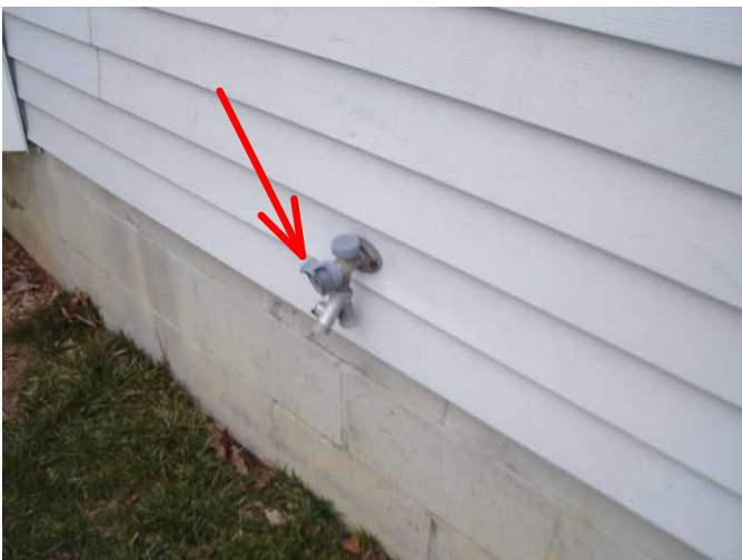
4) Handle on rear hose bib is damaged with sharp edges.
