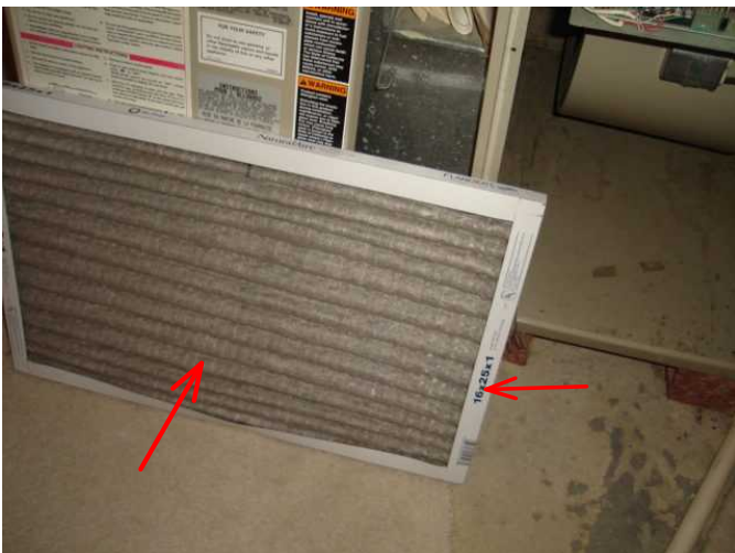
21) Furnace filter dirty. FYI - filter size 16x25x1
