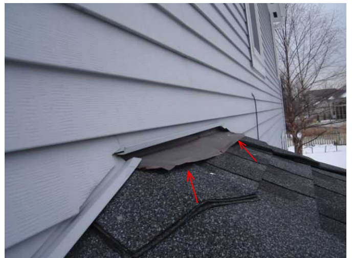
11) Lifted flashing on the rear bay windows
