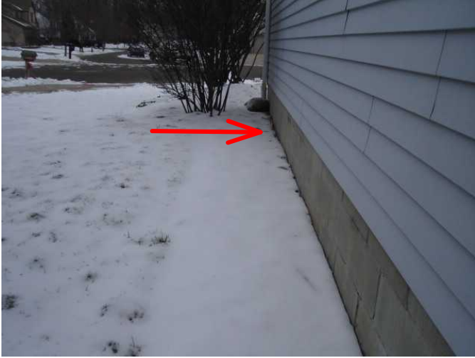
6) Flat to negative grade on west side of structure
