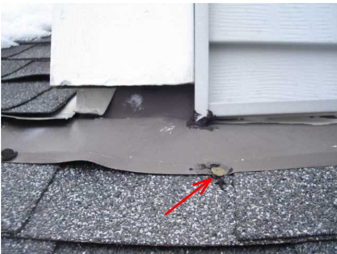
10) Nail head on flashing not sealed and moisture may penetrate to the structure.
