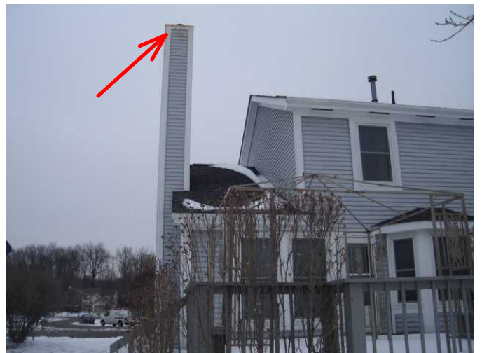
5) Suggest evaluation, cleaning and painting of chimney
