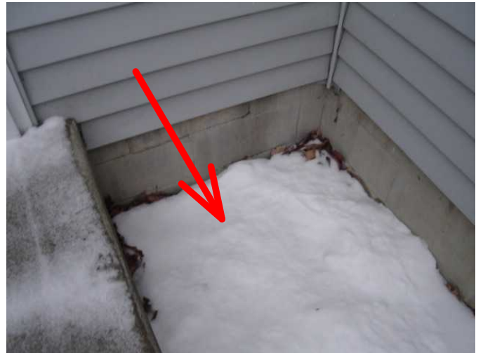
9) Negative grading to right side of front steps. Water will be directed toward the foundation.
