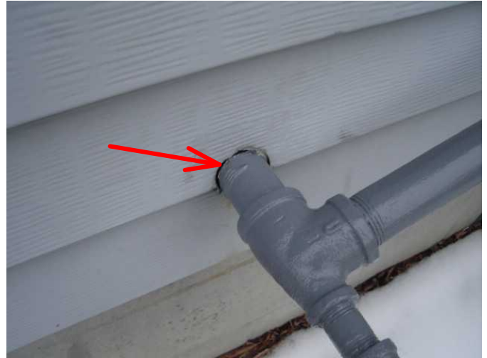
13) Seal at gas meter line entry to the home has deteriorated.
