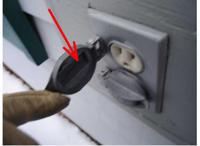
1) Missing weather seal inside front weather proof outlet. Front outlet.
