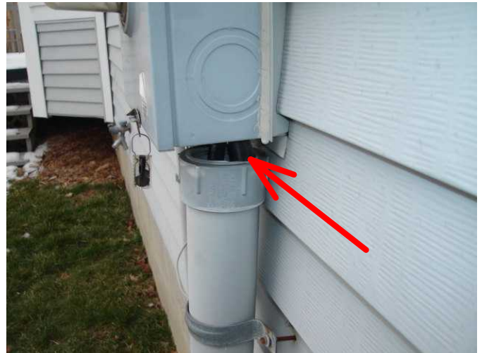
15) Service entry conduit broken at meter box. Pest and moisture may enter the panel. Live wires exposed.
