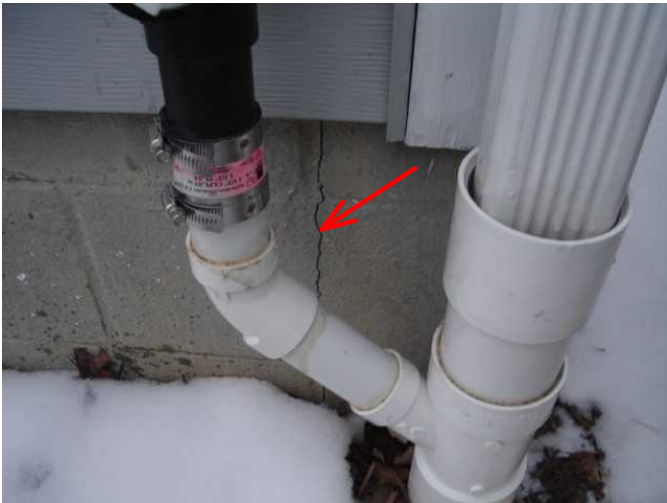
2) One of multiple foundation cracks without displacement. Monitor and repair as needed.
