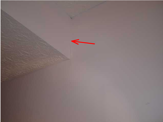
19) Settlement crack in living room / dining room. Repair and monitor.
