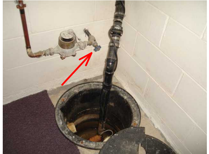
FYI- Main water shut off in basement at sump pump.
