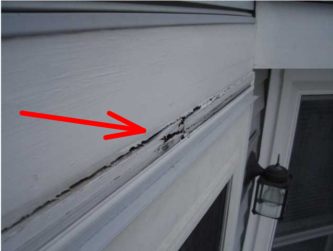
12) Rotten door frame and missing caulk over rear entrance door.
