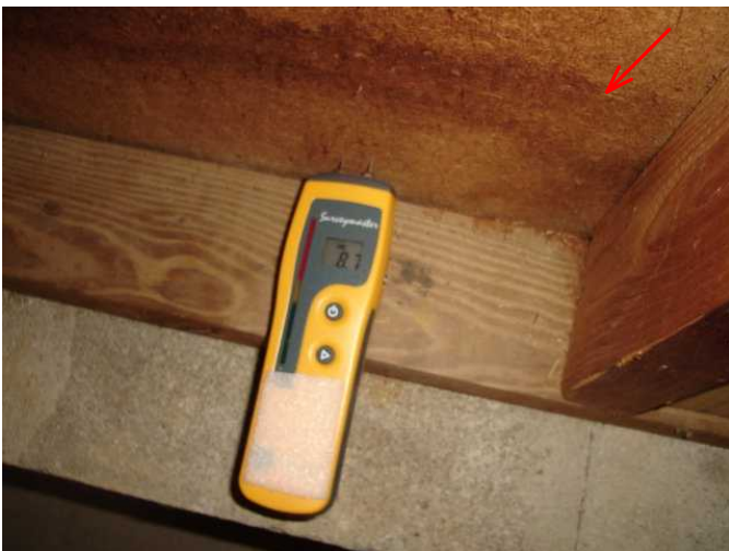
16) Evidence of previous moisture penetration on west garage interior wall. Moisture meter reading of 8.7 percent.
