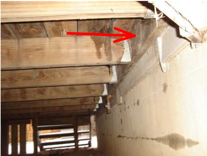
14) Missing lag bolts or through bolts on deck ledger board.
