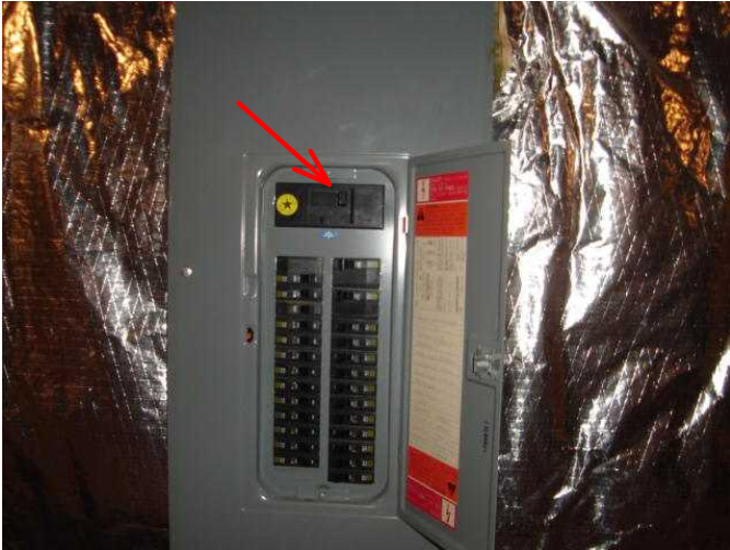
FYI - Main electrical shut off in basement.
