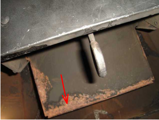
18) Fireplace damper does not stay closed. Evidence of moisture penetration.
