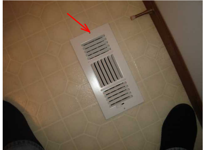
20) Vents in bathrooms are not attached. Safety concern.
