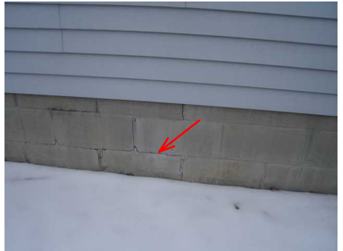
3) Cracks in mortar on foundation.
